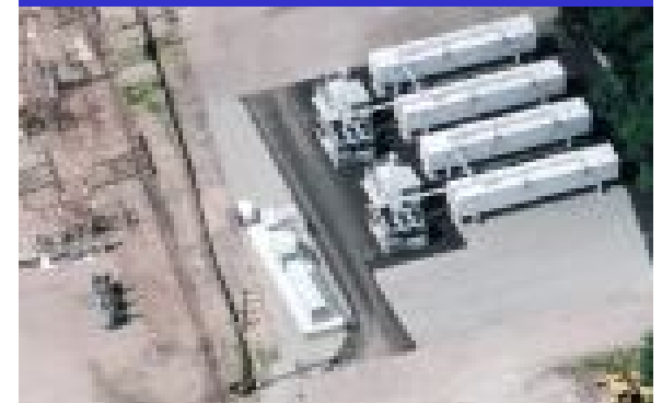
Photo source: AES Energy Storage
